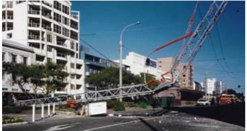
Cambridge Terrace crane collapse
