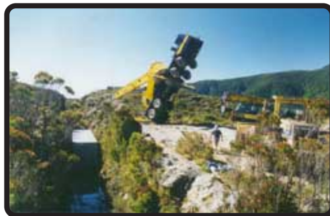
The crane which overturned during the lifting operation.
