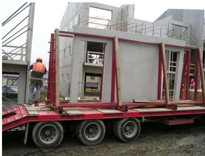
Photo 1: Panels arriving on site with frames showing signs of damage. This method of transportation is common practice in New Zealand.
