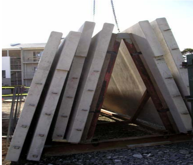
Photo 2: Concrete panels stacked, using current practice, on the frame, as the crane is about to lift it.
